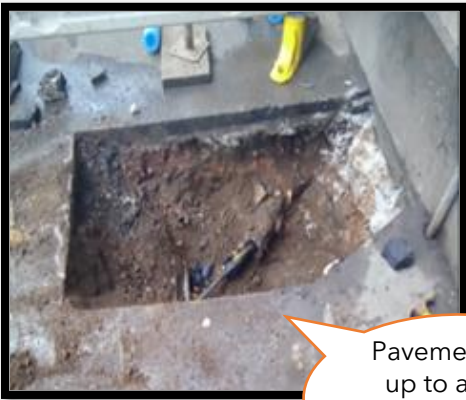
Copper wiring used to illegally re-energise meter
